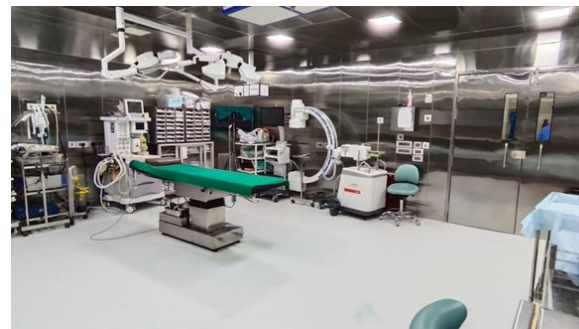
Proposed operating theatre with clean air ventilation, stainless steel walls and anti-static floor.
